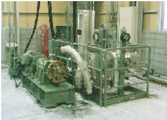
Hot oil test equipment
